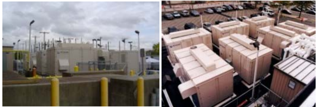
Verizon Fuel Cell Site in Garden City, New York
