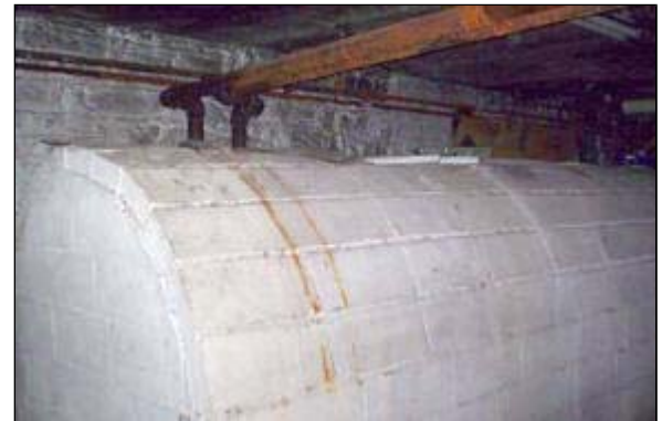
Fuel Oil Tank in Typical Urban Apartment Bldg
